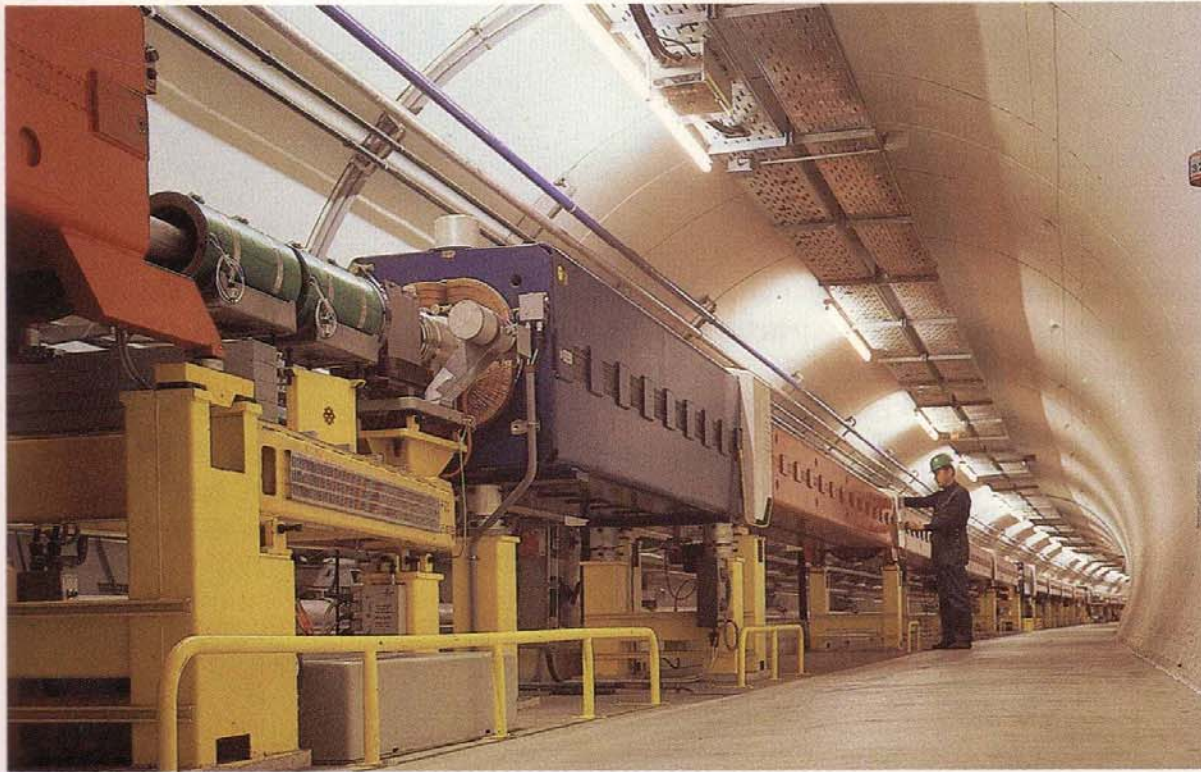
Fig. 8.33 The tunnel of the Super Proton Synchrotron, in the weeks before it accelerated its first protons in 1976. Since 1981 the machine has also operated as a proton-antiproton collider. The same bending magnets (red) and focusing magnets (blue) can guide protons and antiprotons, provided the two types of particle, which have opposite electric charge, are travelling in opposite directions.
